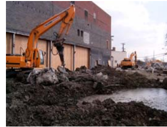
Demolition and removal of existing foundations and buried debris up to 15 feet deep. Extremely soft soils made removal of foundations treacherous since machines would sink while lifting heavy pieces of concrete and debris
