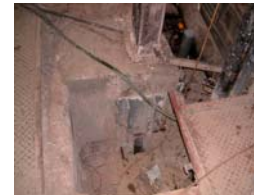
A Micro Pile after installation prior to rerod, grout and cap installation.
