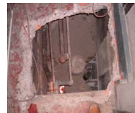
Top down view of a Micro Pile in a concrete utility trench with an active steam line.
