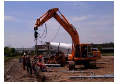
Kent employees installing helical piers in the trench. In the background, the foundation contractor is pouring grade beams.
