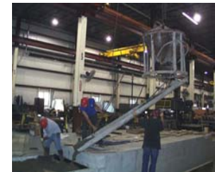
We optimized our resources by engineering a hanging chute for hard to reach areas
